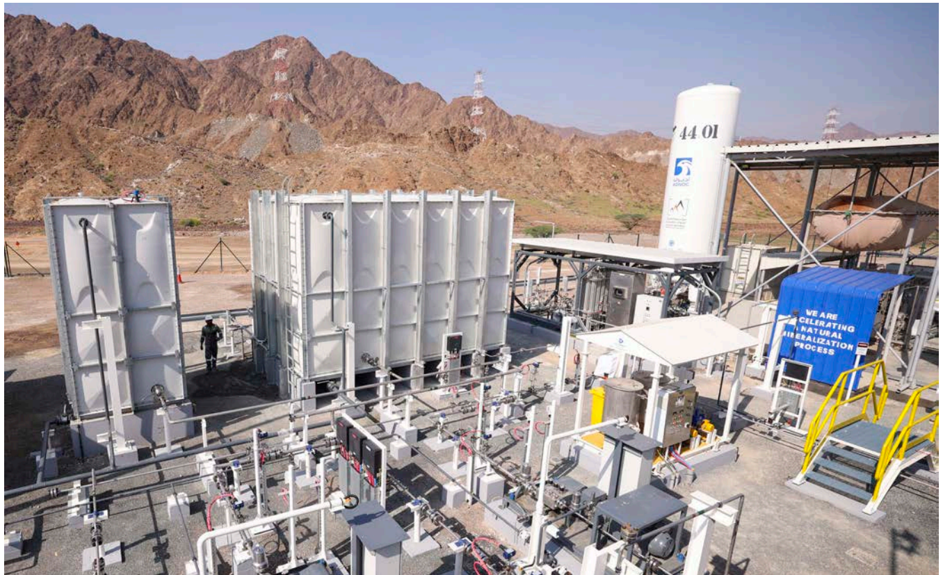
Photo above: A solar-powered ADNOC plant in Fujairah that will, using novel technology, suck carbon dioxide from the air, dissolve it in seawater, and inject it deep underground, where it will mineralize over a period of months. Photo by KARIM SAHIB/AFP via Getty Images.
